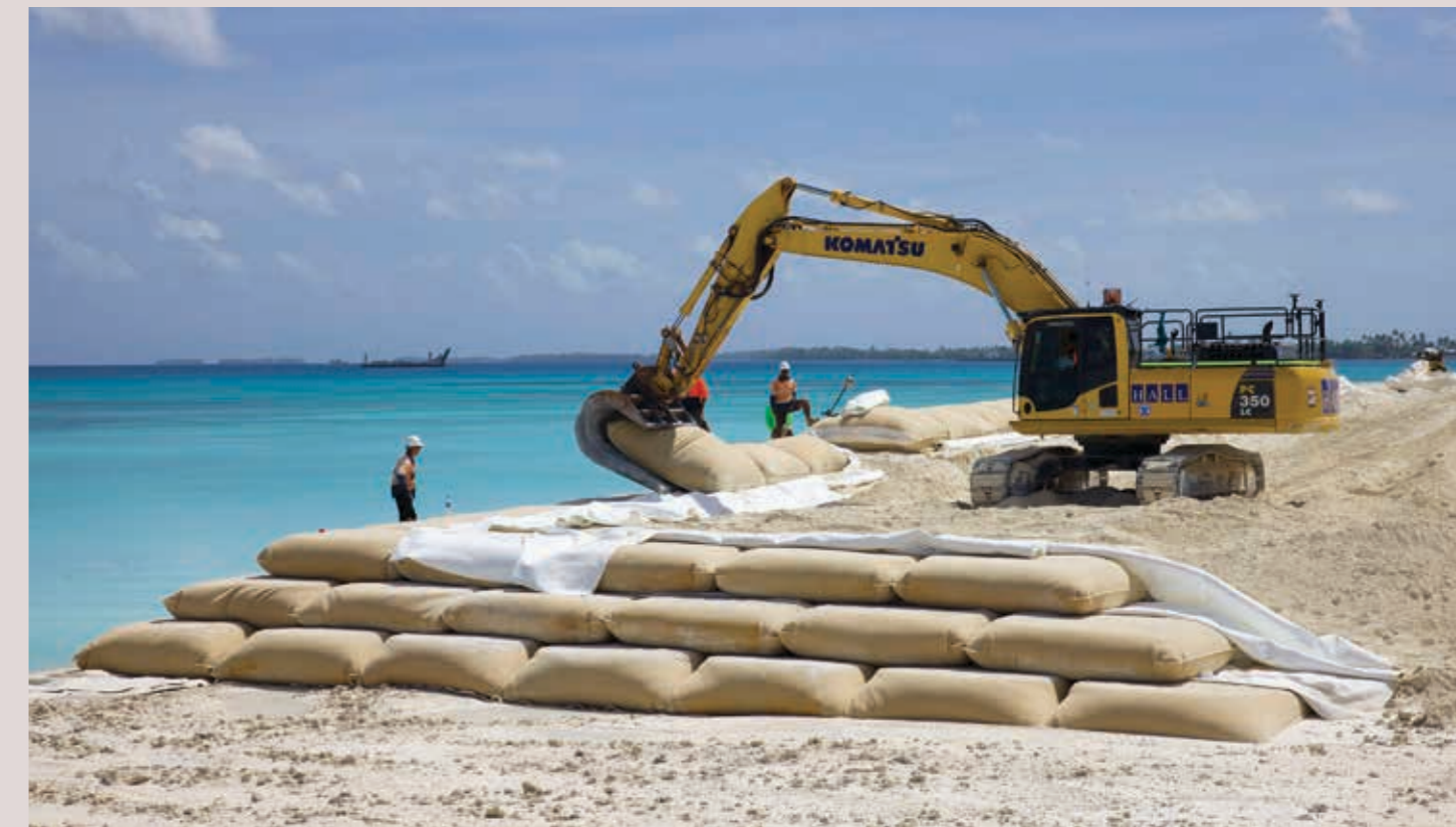
Upgrading the coastal inundation forecast system has enabled customized ocean products for major development projects. © UNDP/TCAP
